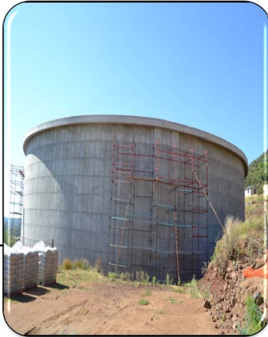
Construction of 15ML Reservoir in Moruleng – Moses Kotane LM at the cost of R25 m
