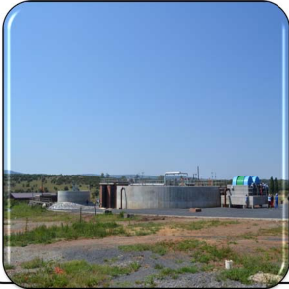
Upgrading of Swartruggens Sewer Treatment Plant – Kgetlengrivier LM at the cost of R26 m
