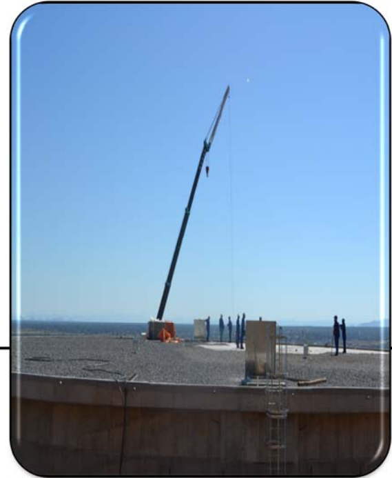
A storage capacity of 15ML Reservoir to supply 48hrs storage in Moruleng area , Moses Kotane local municipality. 21 local people and 2 SMME's were employed during construction.
